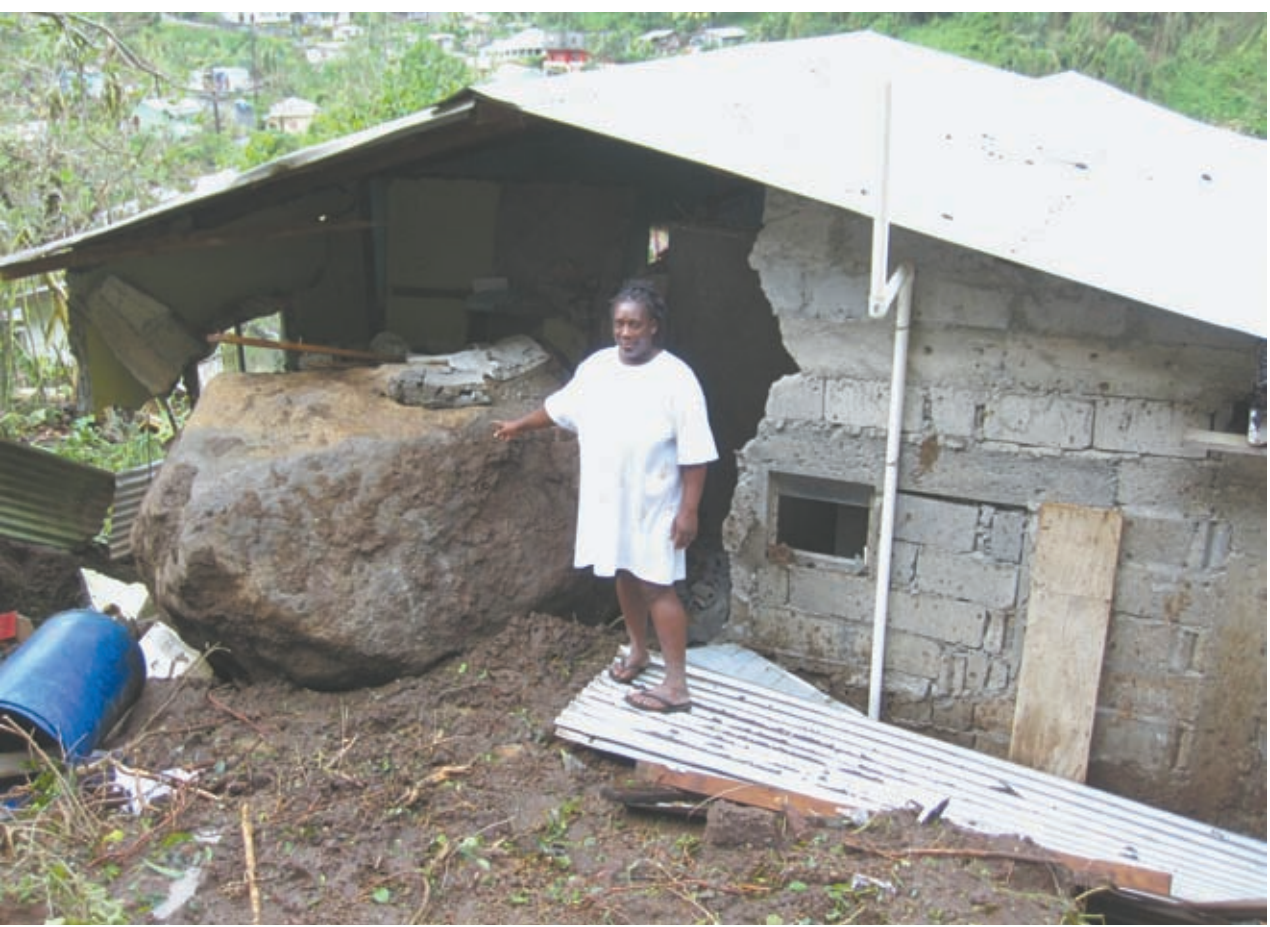
SUSAN ISAACS of Sharpes Village, Chateaubelair, showing the massive boulder that crashed into her home leaving a gaping hole. (See full story on Page 9)
