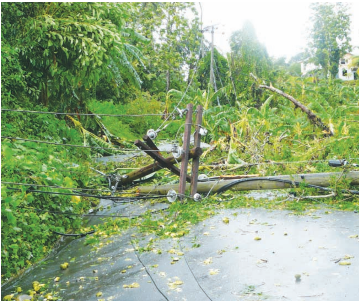
IN PHOTO: Just one of the service lines which fell to the ground after the passing of Hurricane Tomas on Saturday, October 30, 2010.
