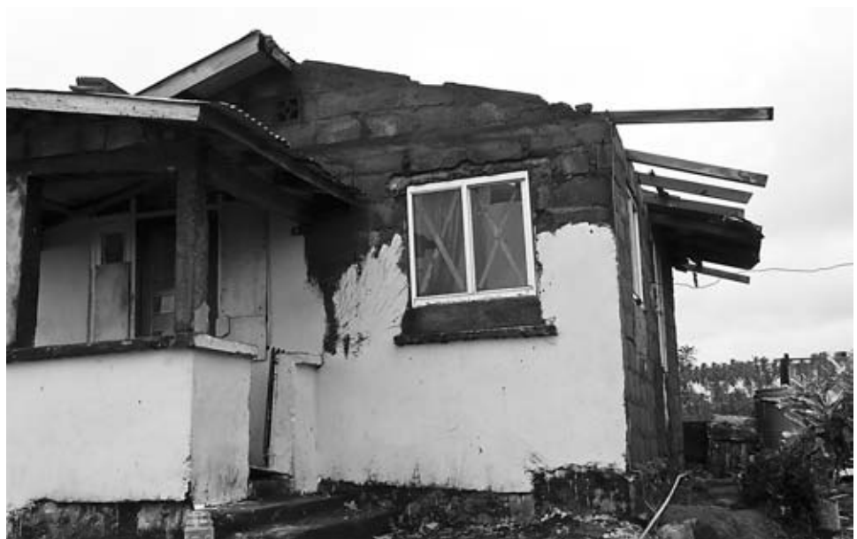
THE REMAINS OF Nanette Cuffy's house that was destroyed during the recent passage of Hurricane Tomas.
