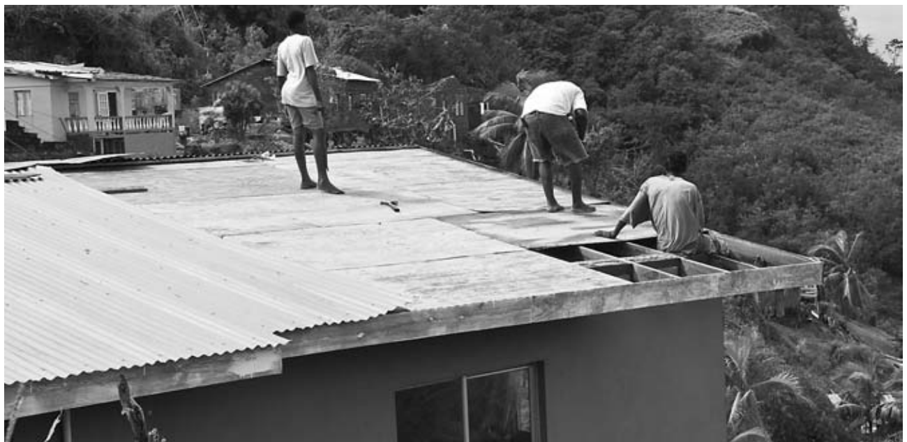
FITZROY BURGESS HOUSE with broken window and roof partially off.
