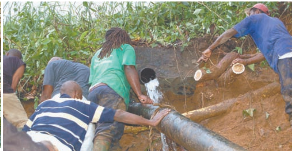
CWSA EMPLOYEES working to repair the broken Majorca main at Riley. Below is the 70ft tree that fell on a section of the Majorca transmission main.
