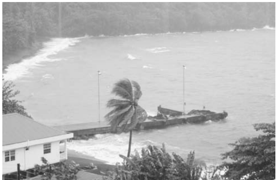
THE CHATEAUBELAIR WHARF taking a sound pounding Saturday morning. It suffered a large crack during the storm.
