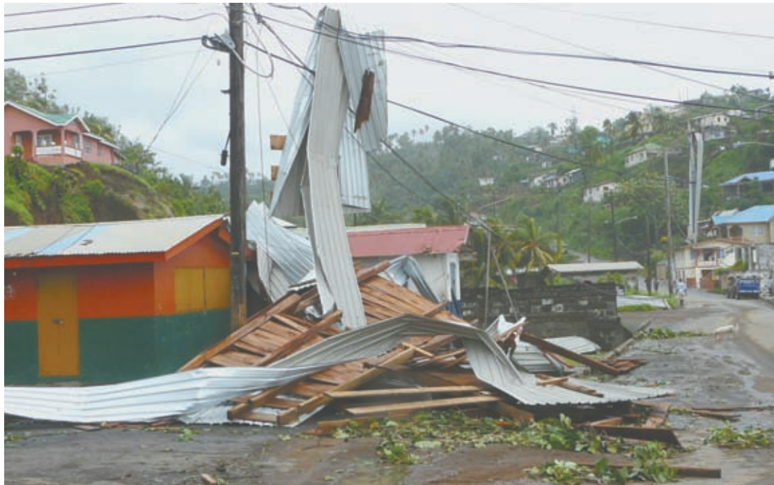
DANGEROUS: Sheets of galvanise were seen wrapped around utility wires.
